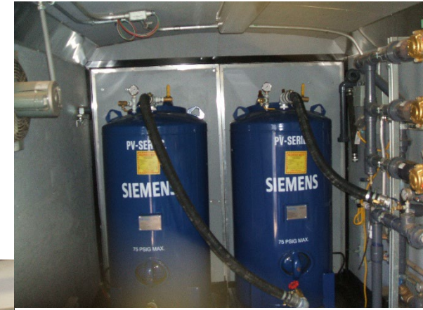
Trailer with GAC Vessels
