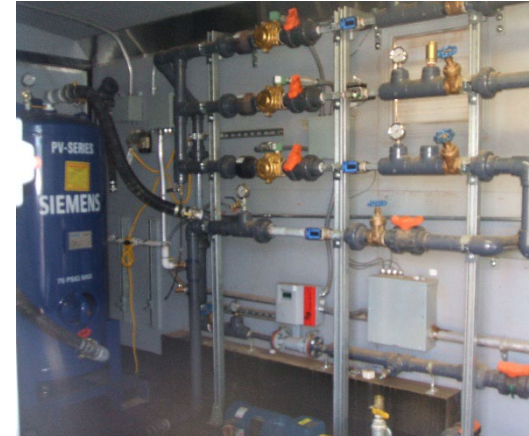
Typical Trailer Manifold System
