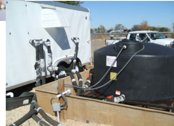
Typical Trailer to EQ Tank
