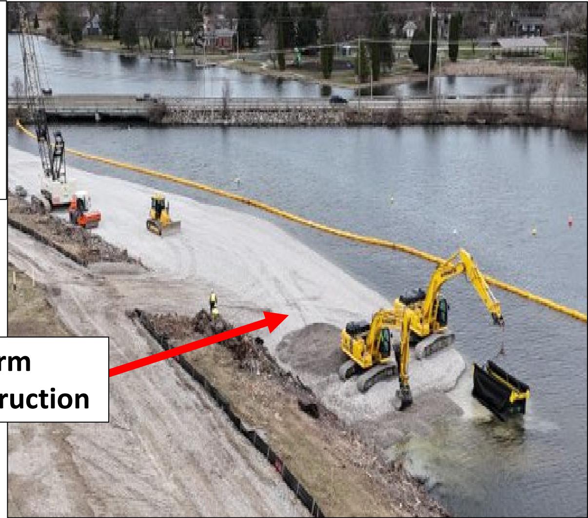
Fabricated tool assists with geotextile installation in the Pine River prior to placement of stone
