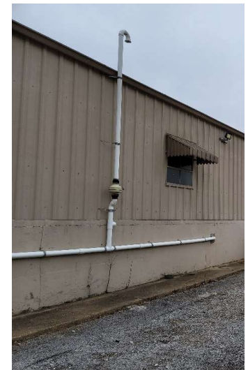
Vapor intrusion mitigation system (VIMS) installed for Walker Building as interim measure
